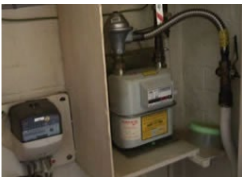
Asbestos panelling around a gas meter
