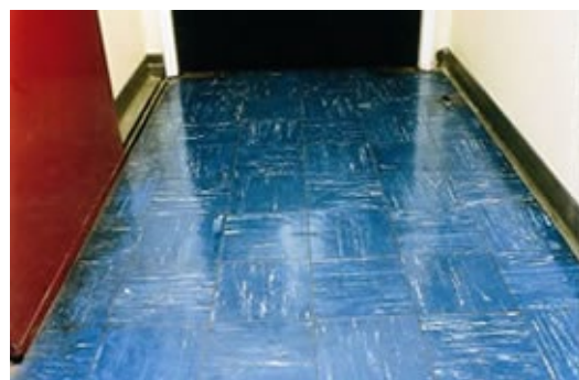
Asbestos containing floor tiles in a corridor
