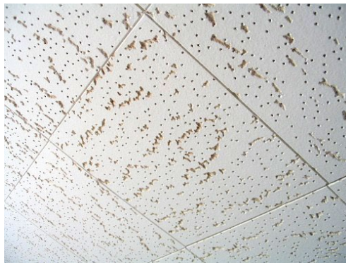
Asbestos containing ceiling tiles
