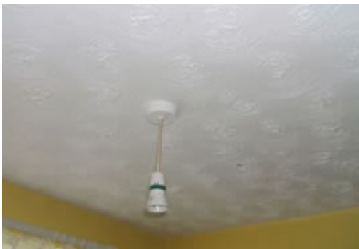
Asbestos textured coating
